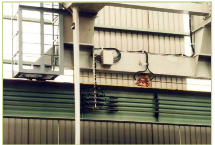
■ POWER SUPPLY FOR THE EDT CRANE AND WELDING EQUIPMENT
