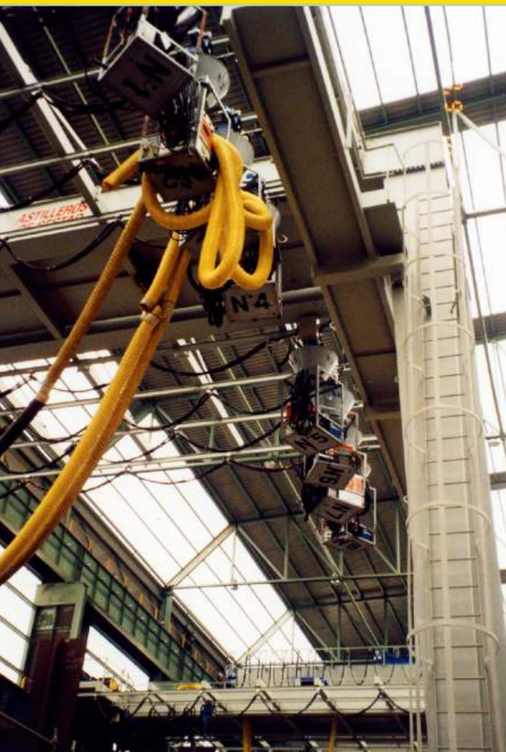
■ SYSTEM FOR THE EXTRACTION OF WELDING GASES
